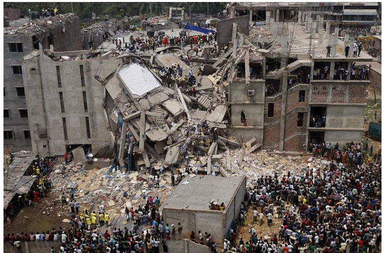
The collapsed Rana Plaza in Bangladesh, where more than 1,100 garment workers were killed. (Wikimedia Commons)
