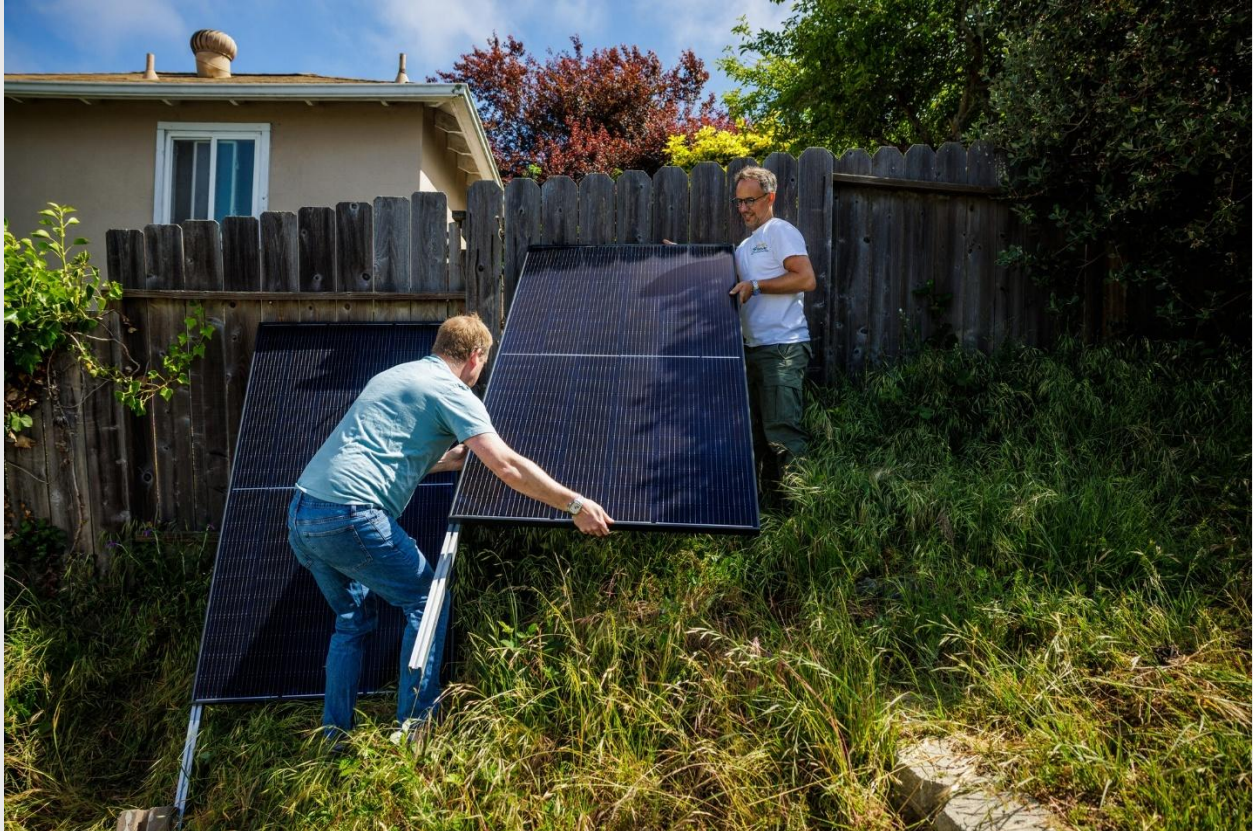
Matthew Milner (left) and Rupert Mayer work to install solar panels in Milner's backyard in Kensington on May 23, 2025.
